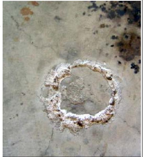
Efflorescence stains on carport floor.
